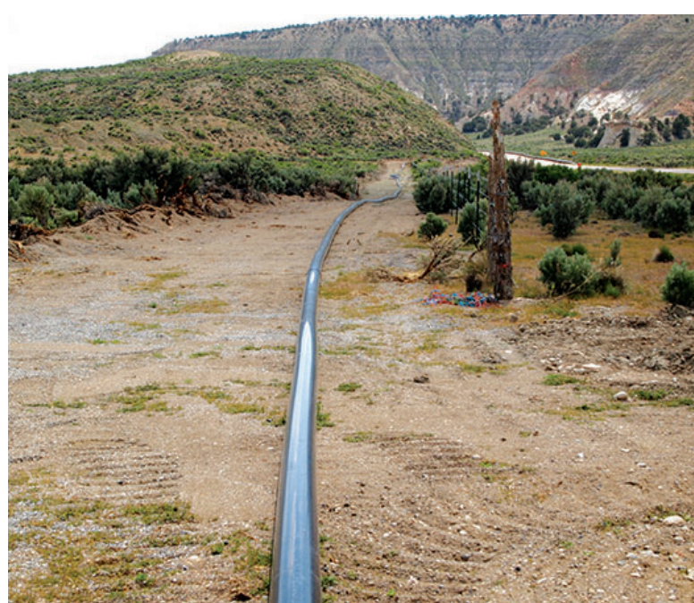
Henrieville's new HDPE culinary water line, awaits trenching along Highway 12 east of Henrieville.
